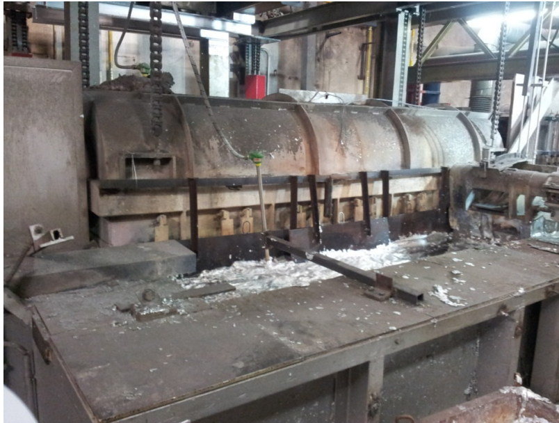
Dip coating system – Zn-Al-Mg
